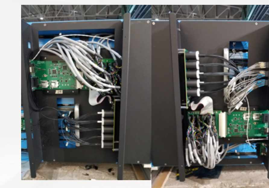
▲ Electronics; power, signal cables; LED drivers and optical fibers
